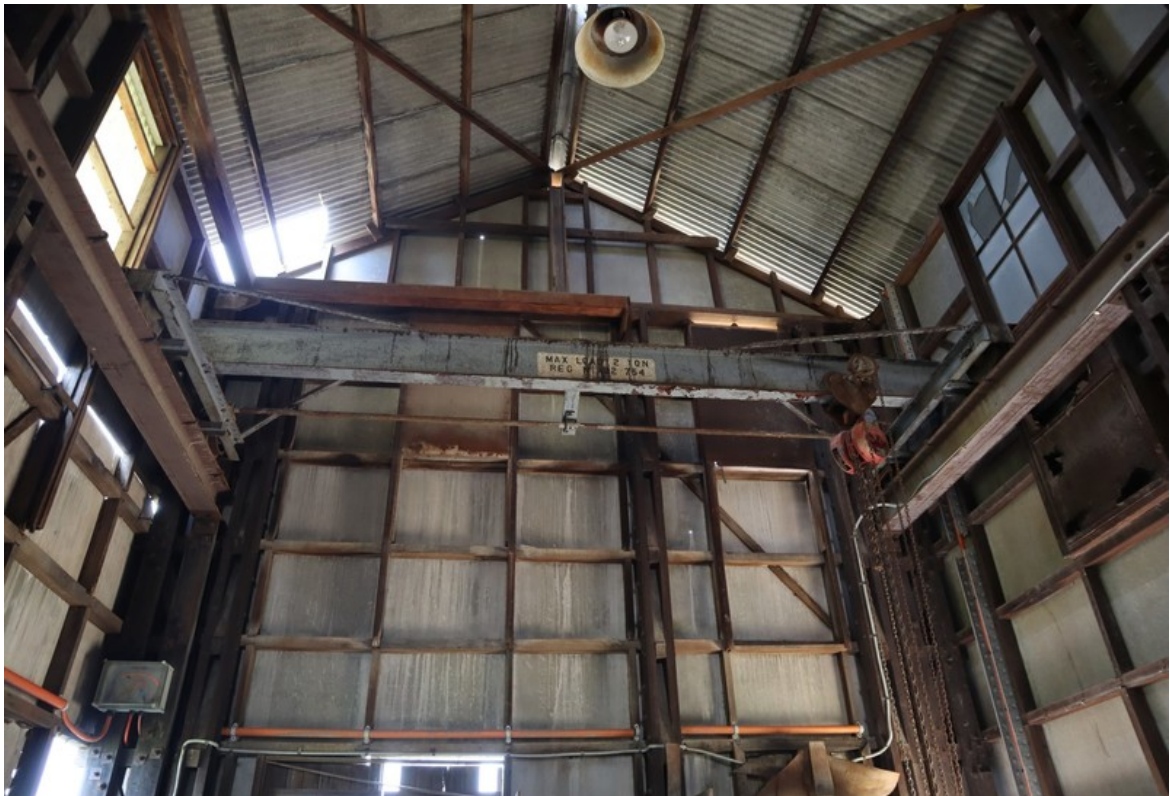
Figure 9: Two ton gantry crane at west end of Base Building (Queensland Government, 2024)
