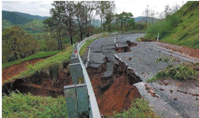
Figure 39: Serious damage around Sarina Range due to landslips from Severe Cyclone Debbie. Source: Loretta MacGregor
