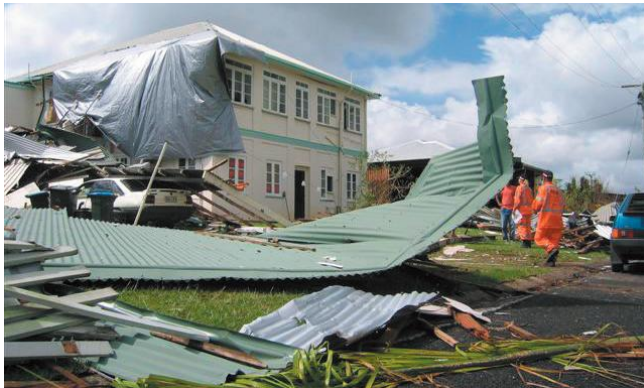
Figure 38: Damage to buildings in Yeppoon in the aftermath of Cyclone Marcia, 2015. Source: Queensland Fire and Emergency Services
