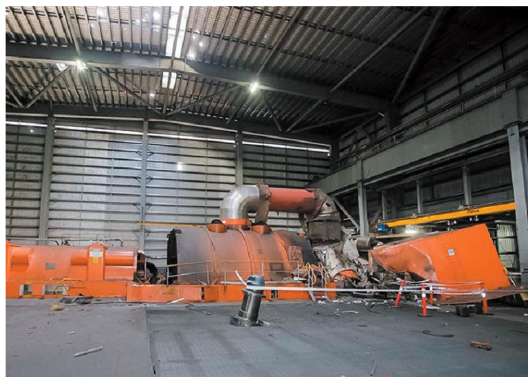
Figure 103: Damage to Unit C4 at Callide Power Station following the plant fire on 25 May, 2021. Source: CS Energy.
