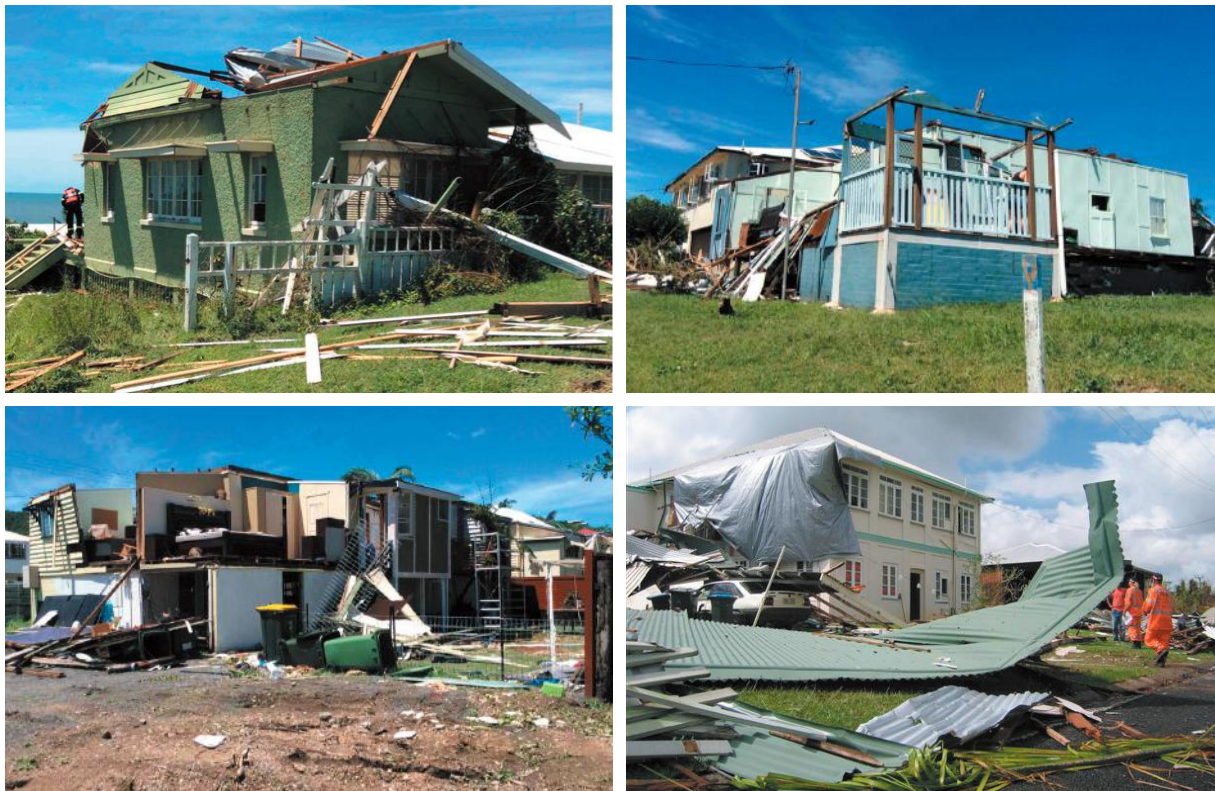
Figure 59: Damage to buildings in Yeppoon in the aftermath of Cyclone Marcia, 2015. Source: Queensland Fire and Emergency Services
